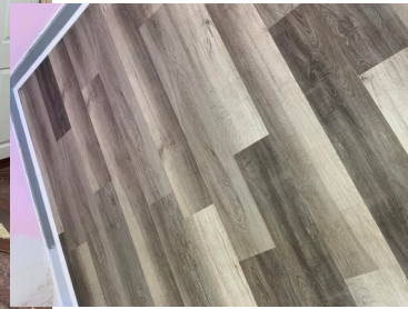
Fixed walls, ceilings, and floor in older dorm, walled in a door & added new flooring
